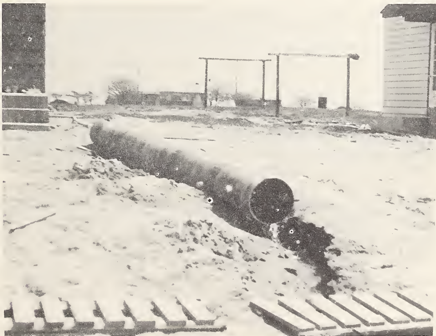
With construction delayed for almost a year by water several feet deep, the owner still planned to build. Construction was started with marsh grass in evidence. (BN-8860-X)
